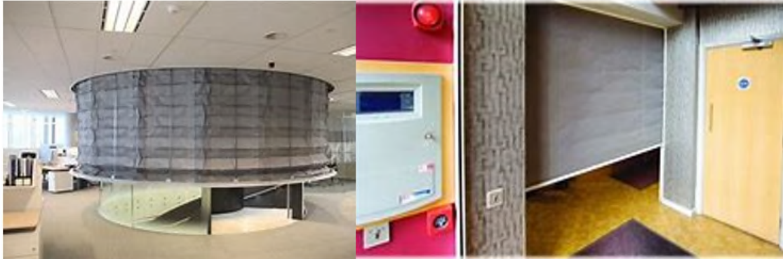
Figure 3: Automatic Fire Barriers
